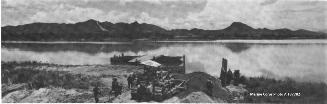
Figure: Original caption: Marine engineers work on the extension for Liberty Road to An Hoa. The troops are laying down abutments for a pontoon ferry which will link An Hoa to Da Nang.
